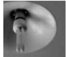
An example Compact Fluorescent Light bulb replacing a fitting that formerly held an incandescent.
